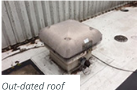
Out-dated roof extract unit
