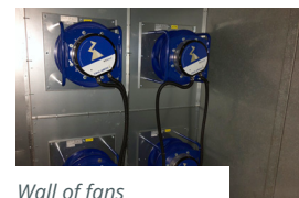
Wall of fans
