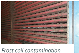
Frost coil contamination
